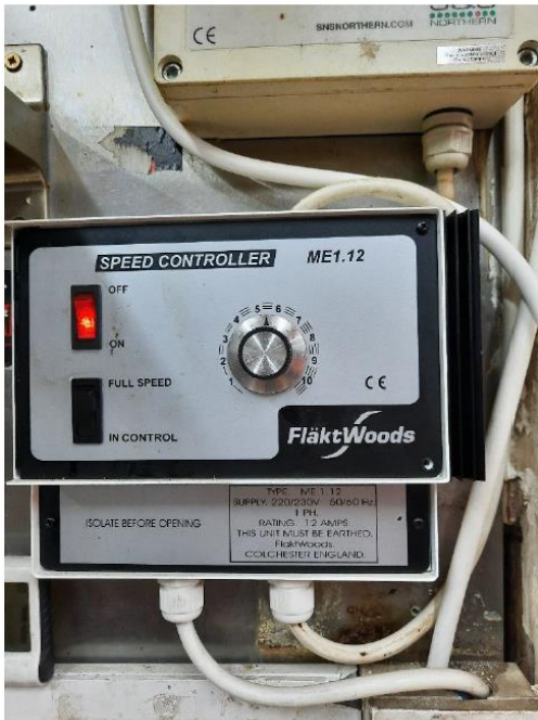
Figure 4: Fan speed controller at correct setting
