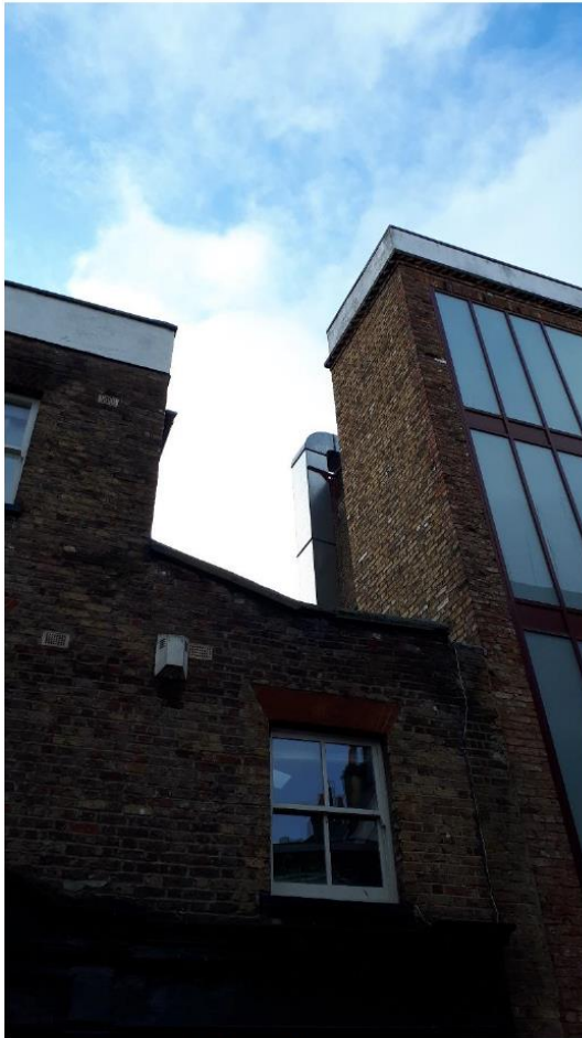
Figure 2: Extract ducting to the rear
