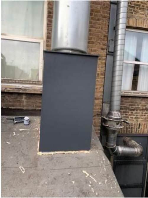
Figure 3: Acoustic enclosure around fan
